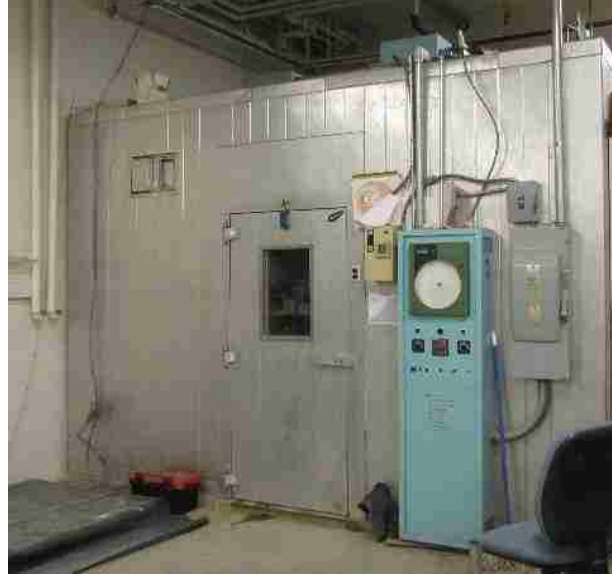
Figure 5. Environmental test chamber
