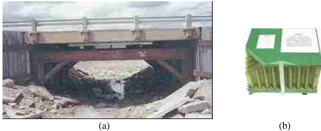
Figure 2.3. The no-name creek bridge in Russell, KS (a) Bridge overview and (b) Honeycomb core
